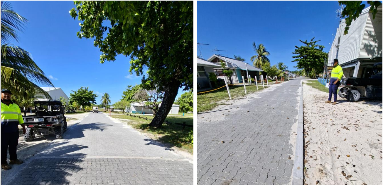
Figure 4: Sections of road paving was replaced and broken concrete edge strips were repaired on streets on Home Island.
