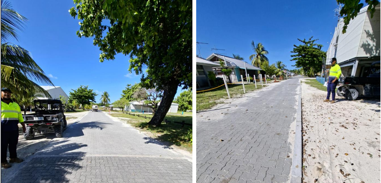
Figure 4: Sections of road paving was replaced and broken concrete edge strips were repaired on streets on Home Island.
