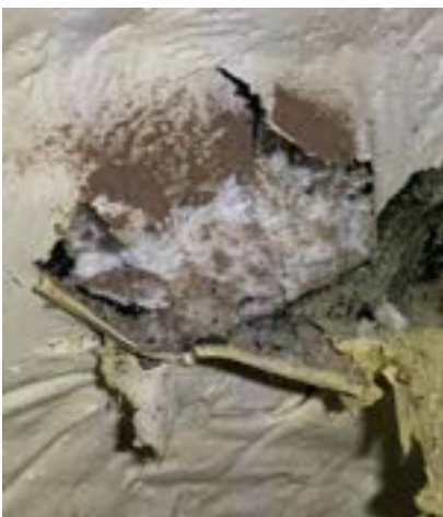
Salt Deposit underneath paint
