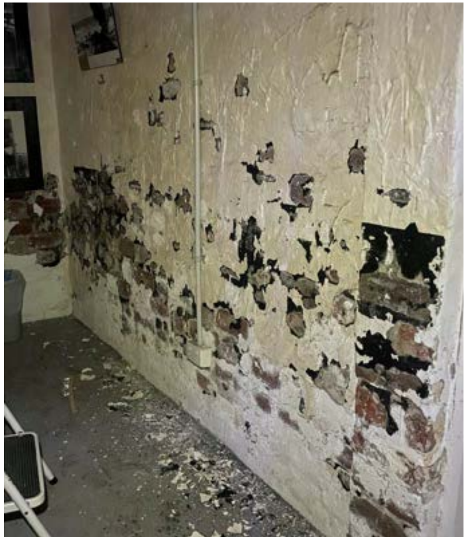
Salt Deposits removed from a section of wall
