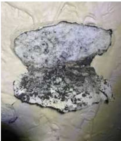
Salt Deposit underneath paint
