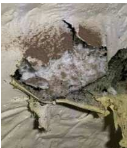
Salt Deposit underneath paint
